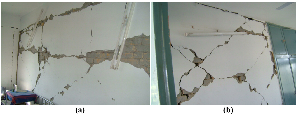
Figure 4: (a) Flexural & shear cracks alongwith separation of wall from wall connection (b) Shear & flexural cracks alongwith separation of wall from roof
