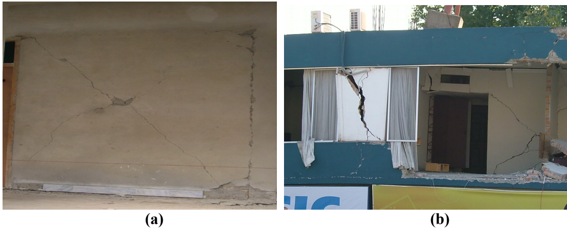
Figure 3: (a) Shear cracks in masonry load bearing wall (Muzaffrabad University) (b) Shear cracks in masonry infill in shopping plaza at Abbottabad
